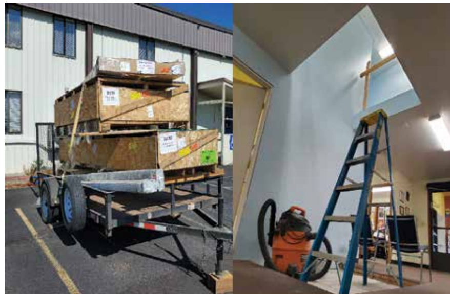
Construction Update! The elevator was delivered on May 30. Pictured LEFT is the elevator awaiting assembly. RIGHT is downstairs, looking up to the 2nd floor where the elevator will be installed - which will likely be by the time you read this!
